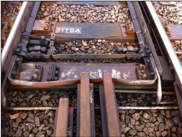
Damaged stretcher bar
