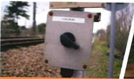
Example of a TOWS switch
